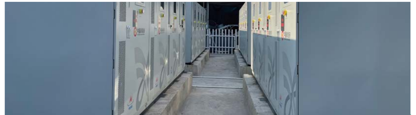
Zhejiang Limin User Side Energy Storage Power Station Project
