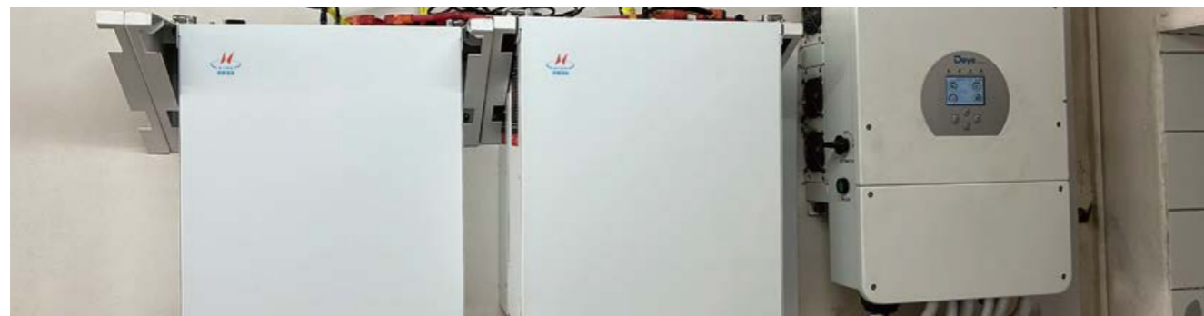
Johannesburg area (residential energy storage batteries)
