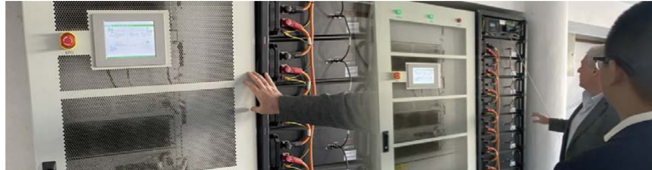
C&I Energy Storage in Italy
